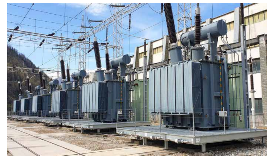
Valpelline power plant: on-line DGA monitoring of the 6 single-phase transformers
